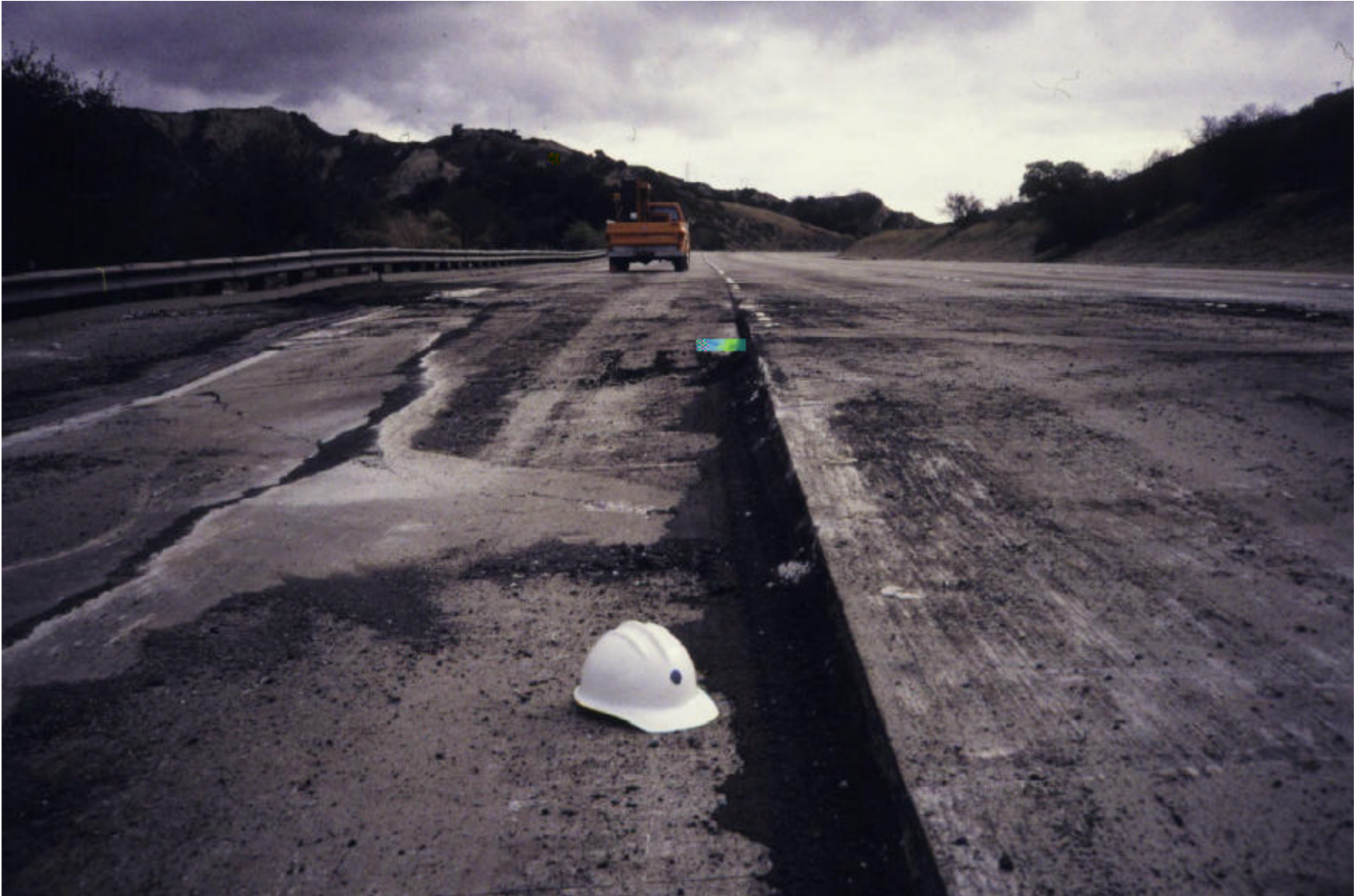
15 Near Gavin Canyon, 1994 Northridge Earthquake (M.O. Eberhard)
