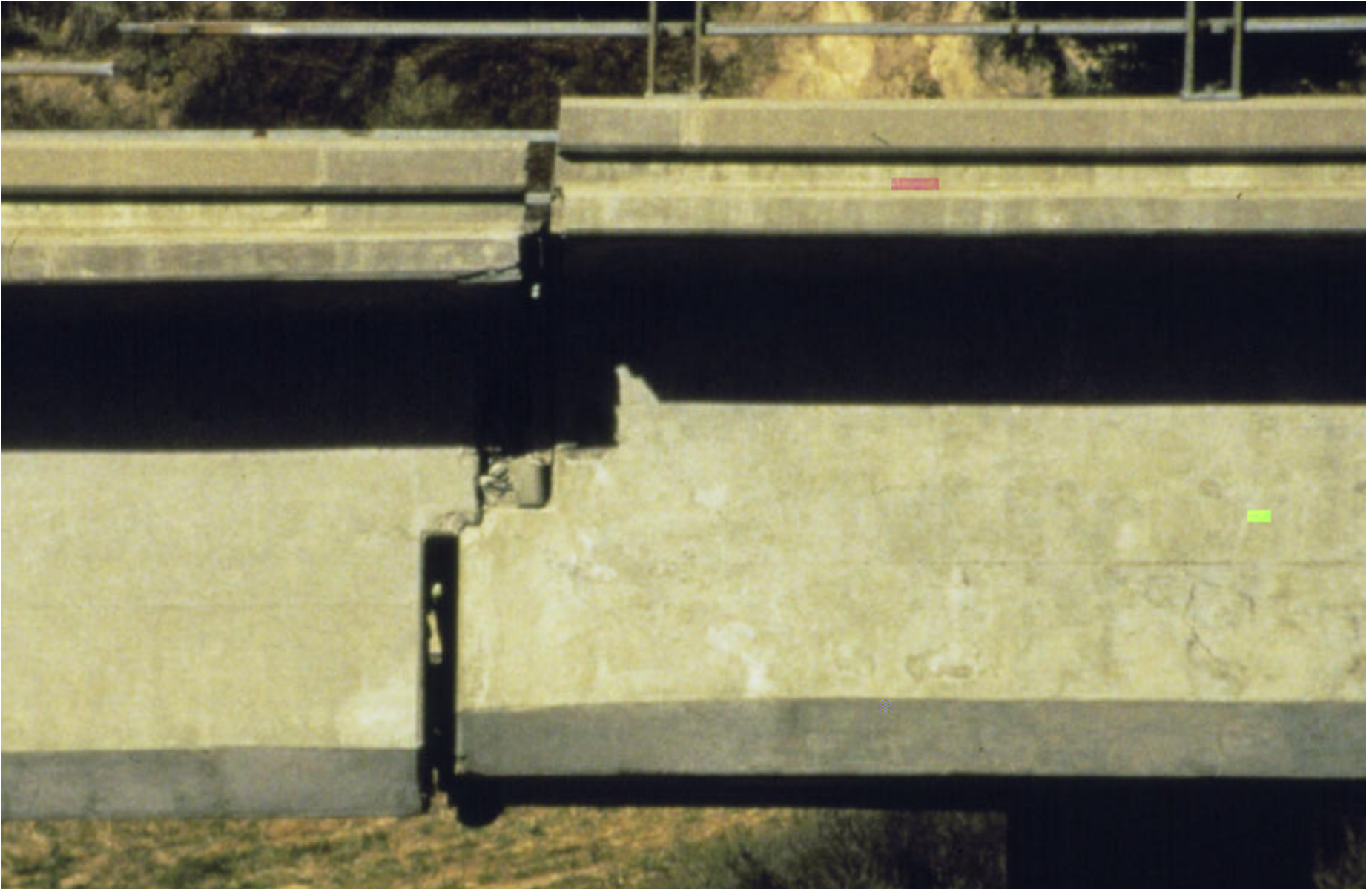
I5-14 Interchange, 1994 Northridge Earthquake (M.O. Eberhard)
