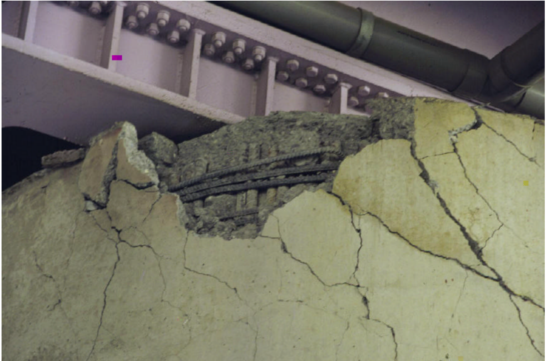
Mhau-Luo-Shi Bridge, 1999 Chi-Chi Eq. (M.O. Eberhard)
