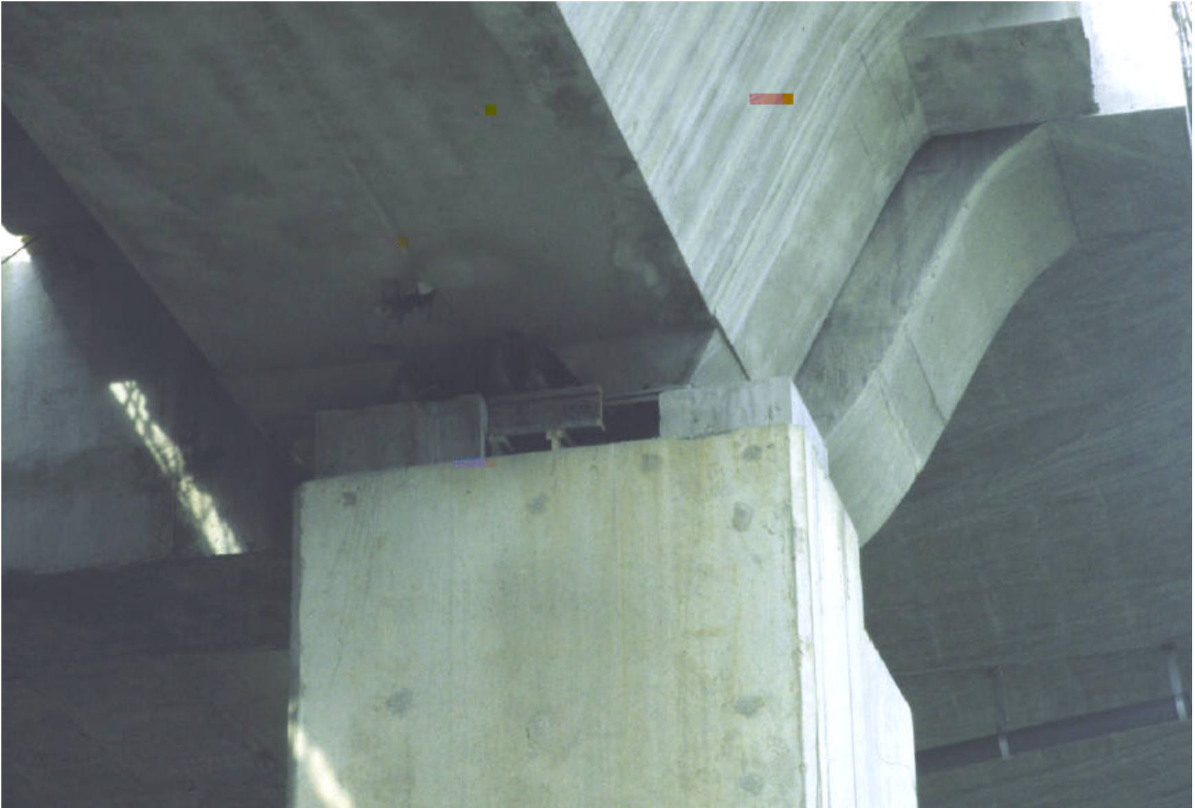
1-3 Expressway Link, 1999 Chi-Chi Eq. (M.O. Eberhard)
