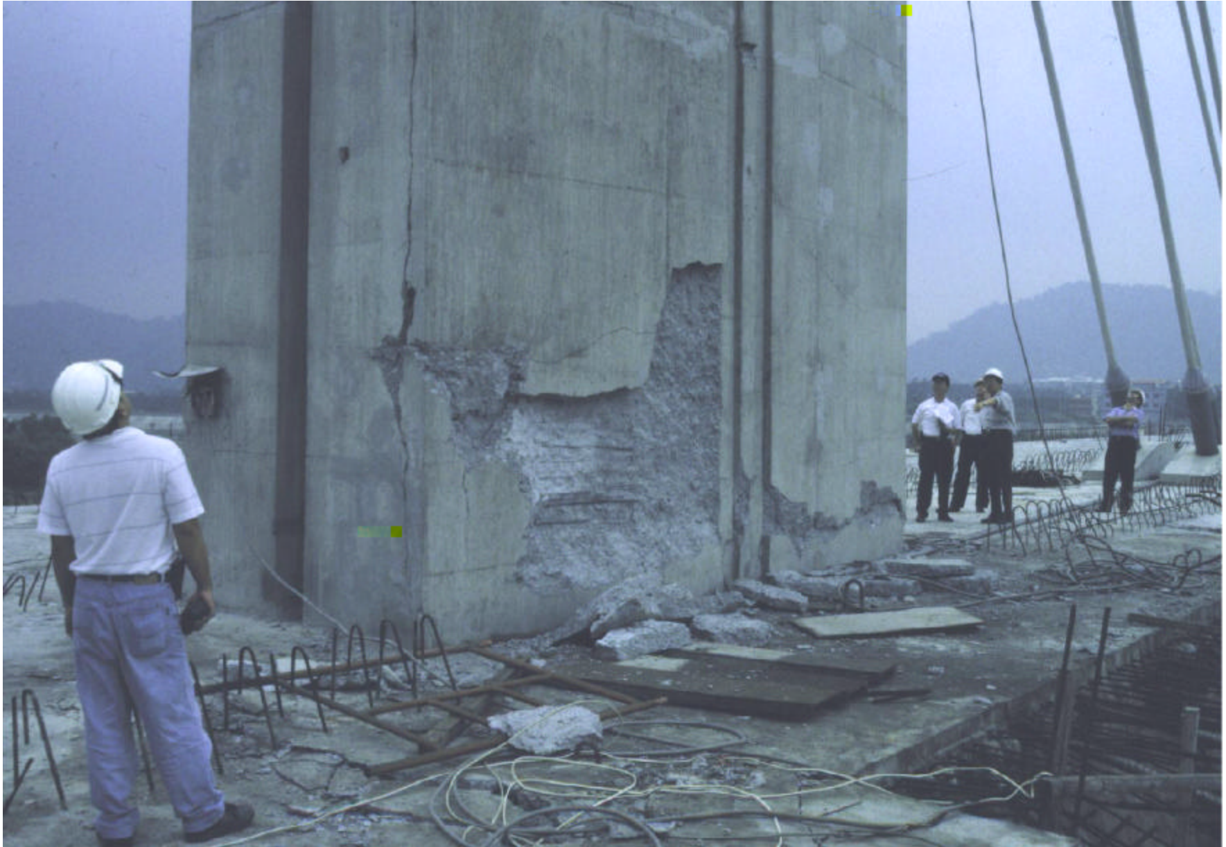
Cable-Stayed Bridge, 1999 Chi-Chi Eq. (M.O. Eberhard)
