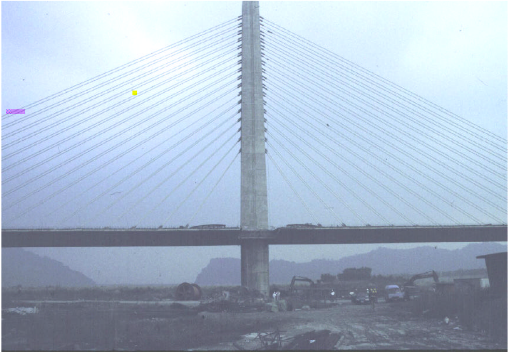
Cable-Stayed Bridge, 1999 Chi-Chi Eq. (M.O. Eberhard)
