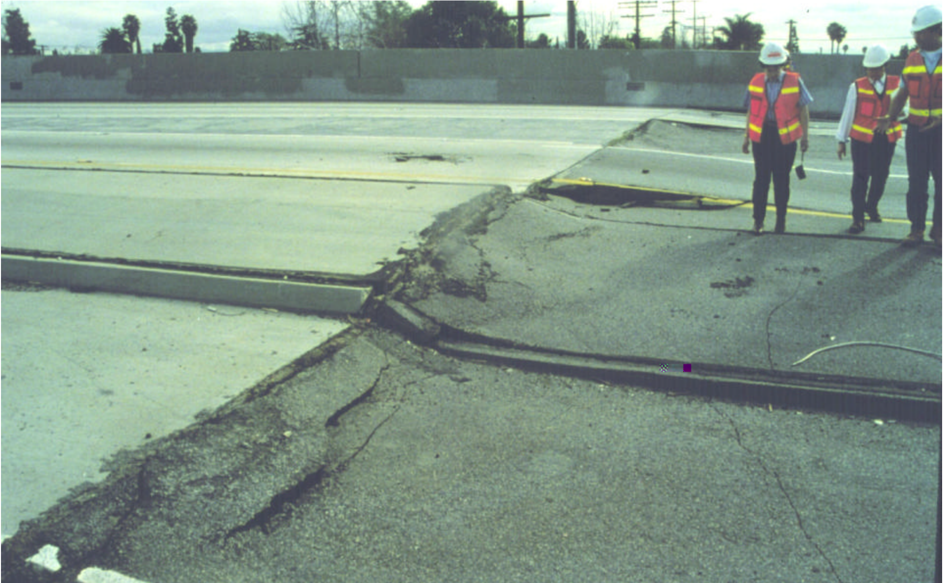
I-118, 1994 Northridge Earthquake (M.O. Eberhard)
