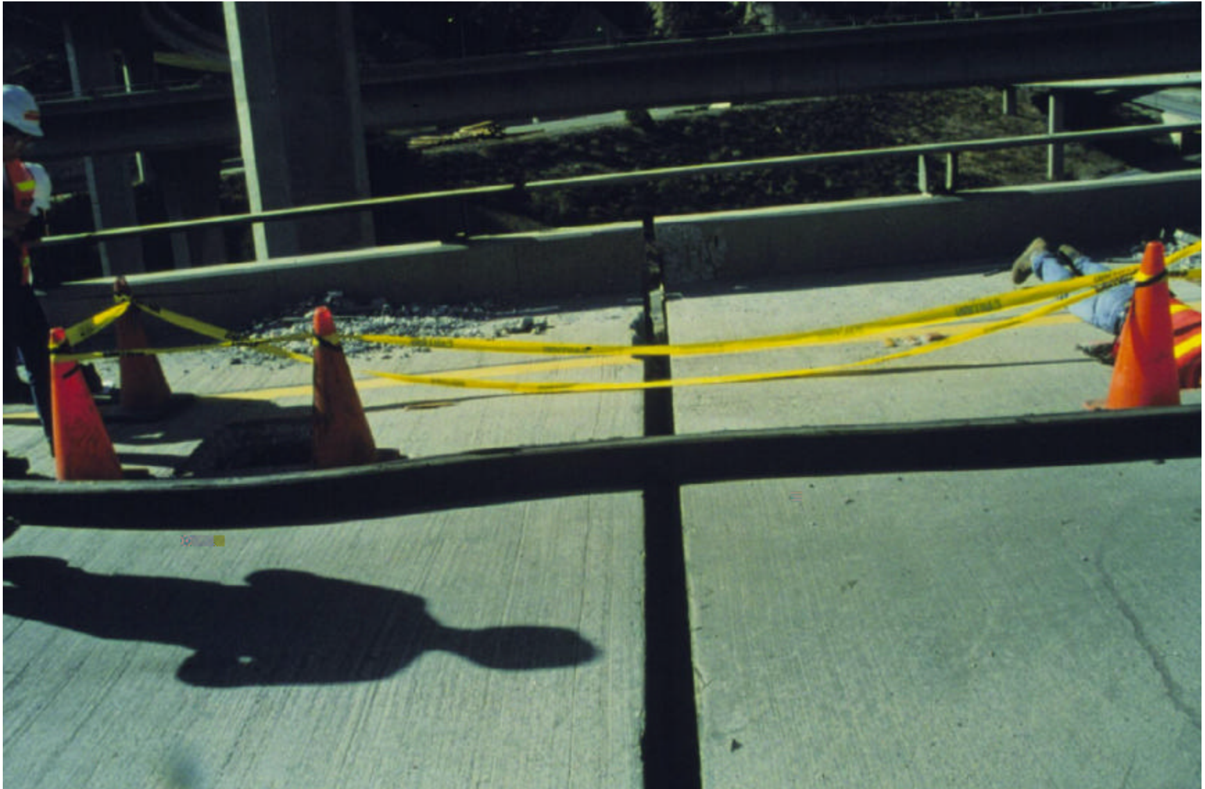
15-14, 1994 Northridge Earthquake (M.O. Eberhard)
