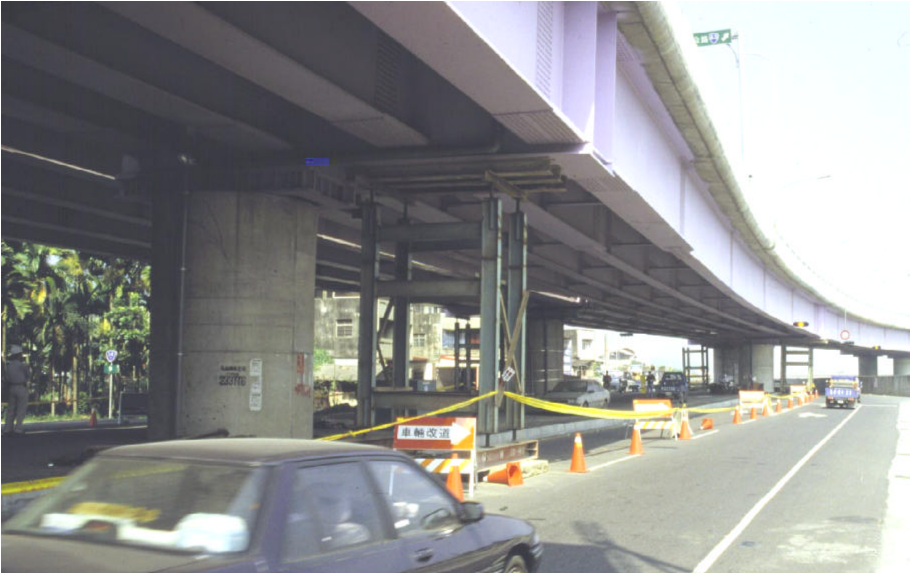
Mhau-Luo-Shi Bridge, 1999 Chi-Chi Eq. (M.O. Eberhard)
