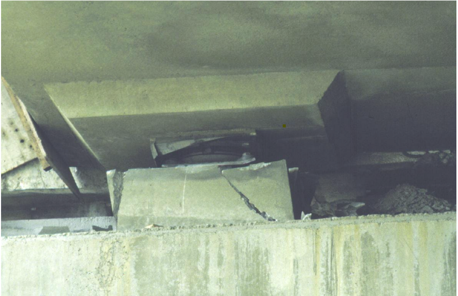
1-3 Expressway Link, 1999 Chi-Chi Eq. (M.O. Eberhard)
