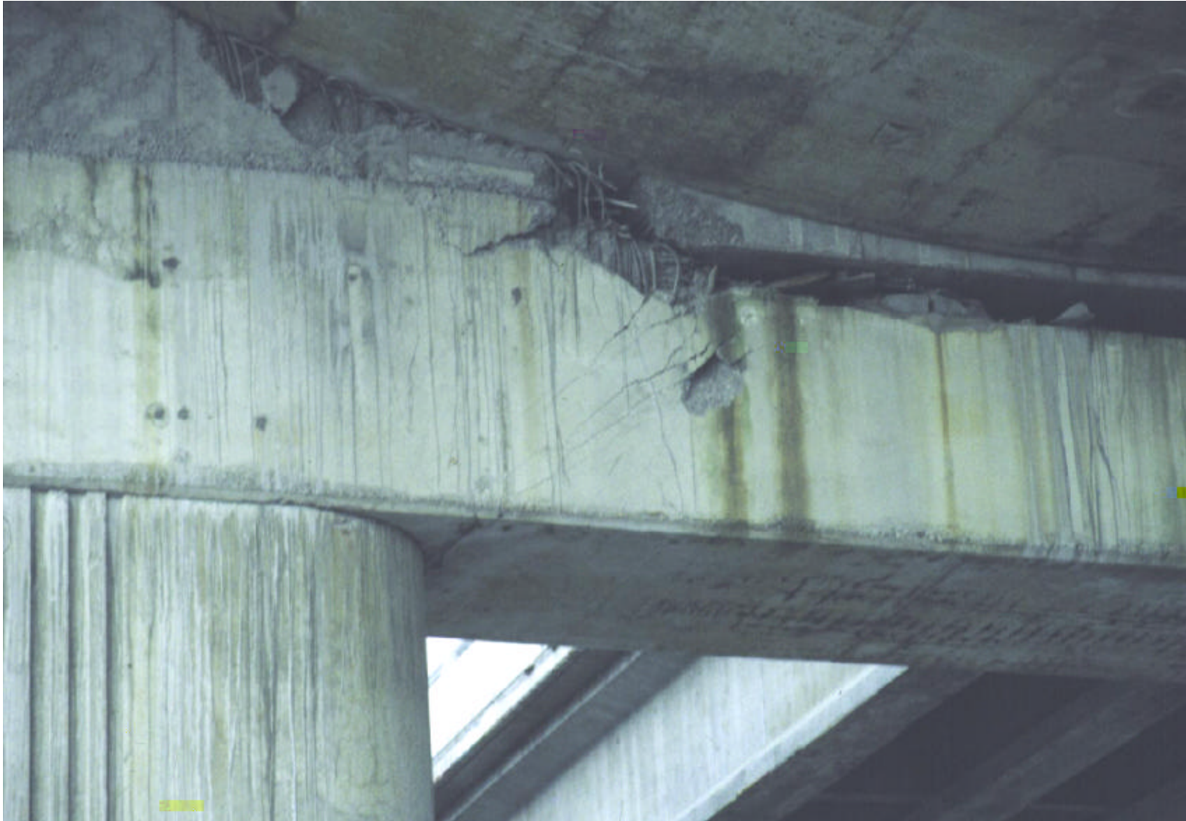
Cable-Stayed Bridge, 1999 Chi-Chi Eq. (M.O. Eberhard)
