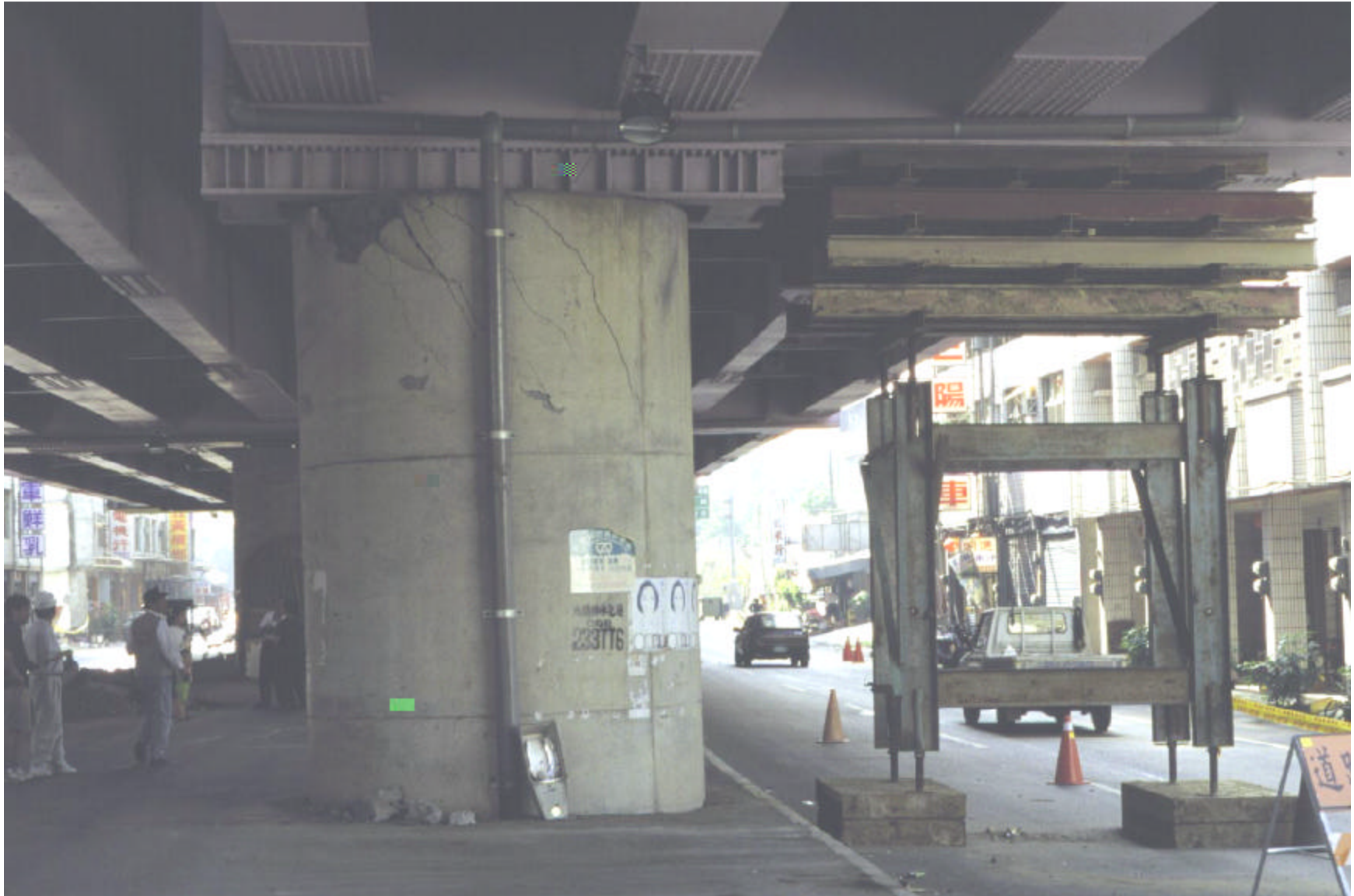
Mhau-Luo-Shi Bridge, 1999 Chi-Chi Eq. (M.O. Eberhard)
