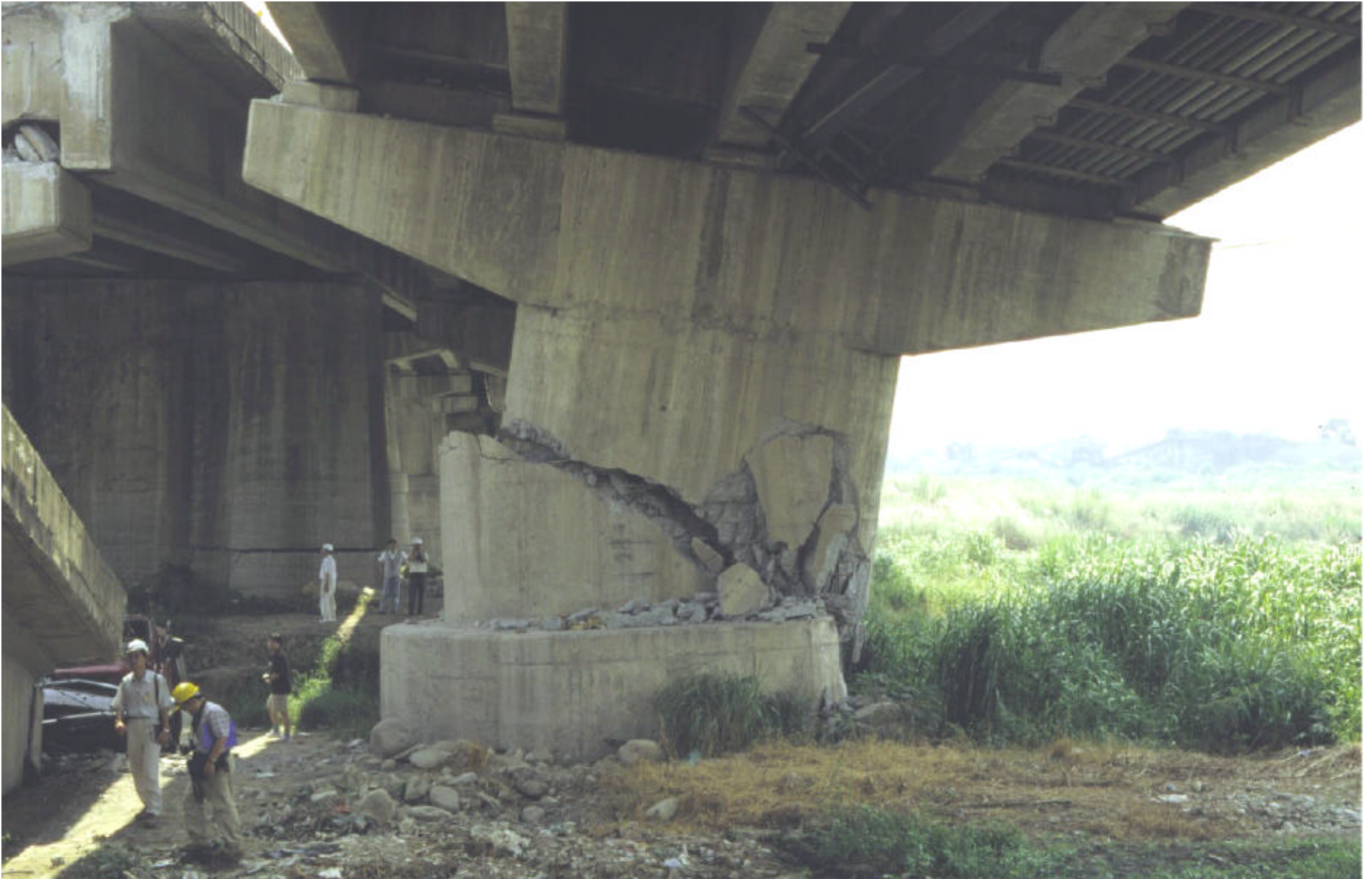
U-Shi Bridge, 1999 Chi-Chi Eq. (M.O. Eberhard)
