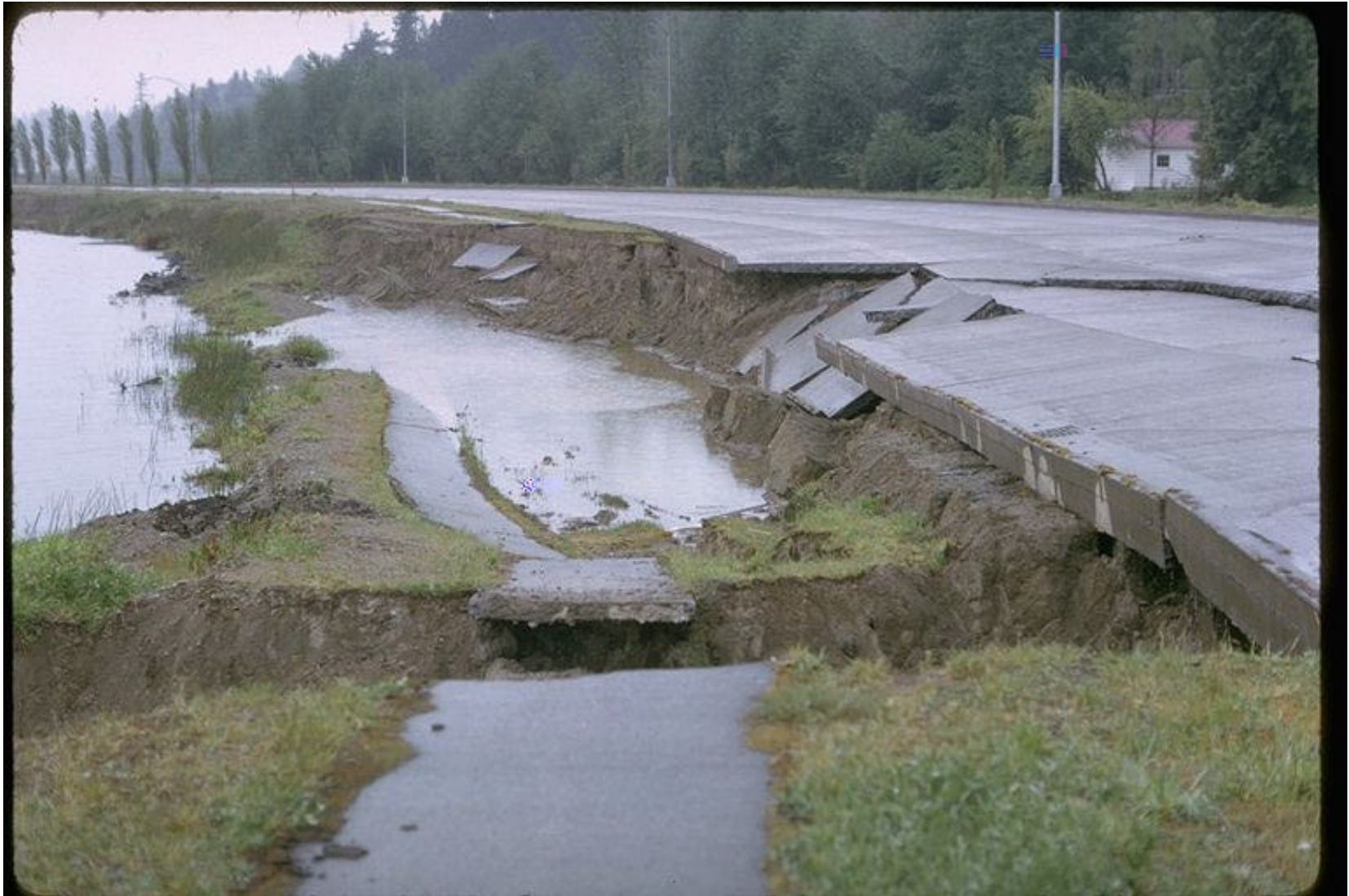
Puget Sound Earthquake, 1965. (Steinbrugge Collection, EERC)
