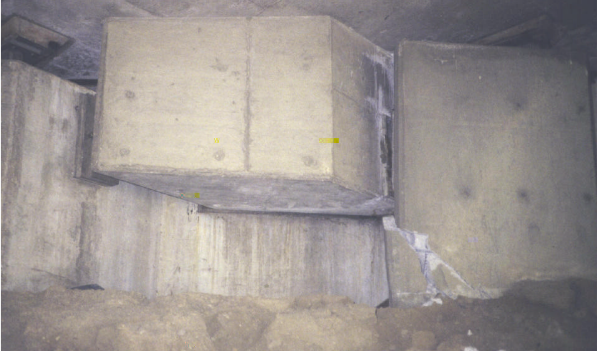
I5-14 Interchange, 1994 Northridge Earthquake (M.O. Eberhard)
