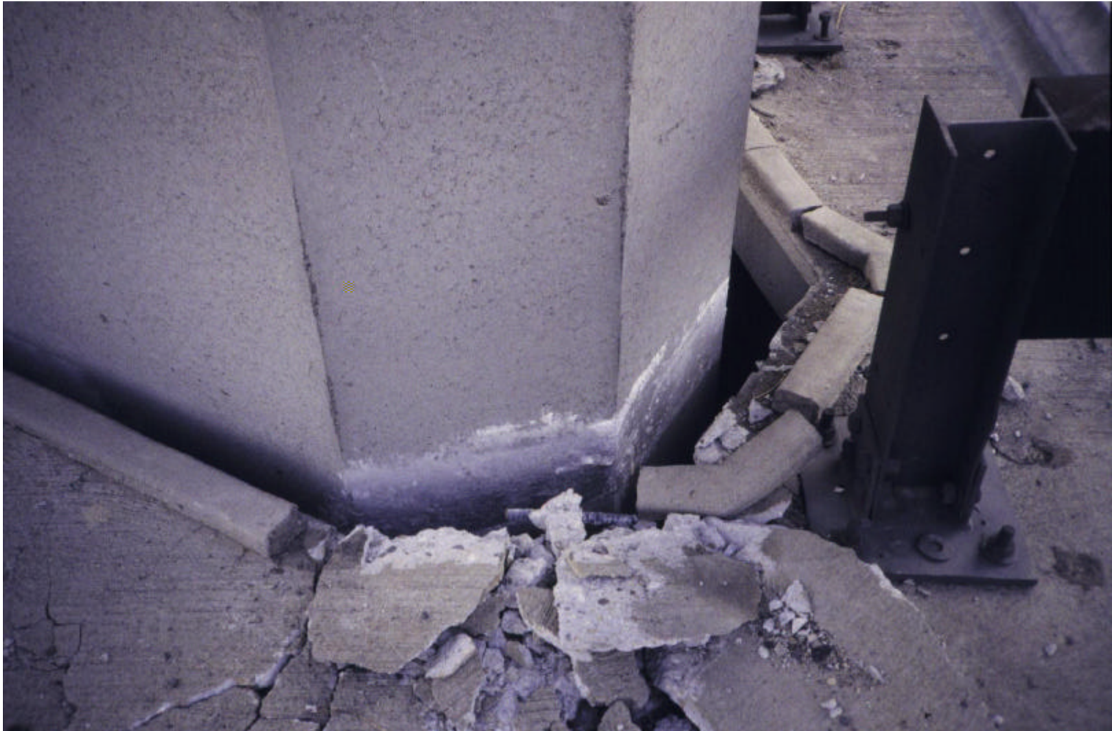
I5-210, 1994 Northridge Earthquake (M.O. Eberhard)
