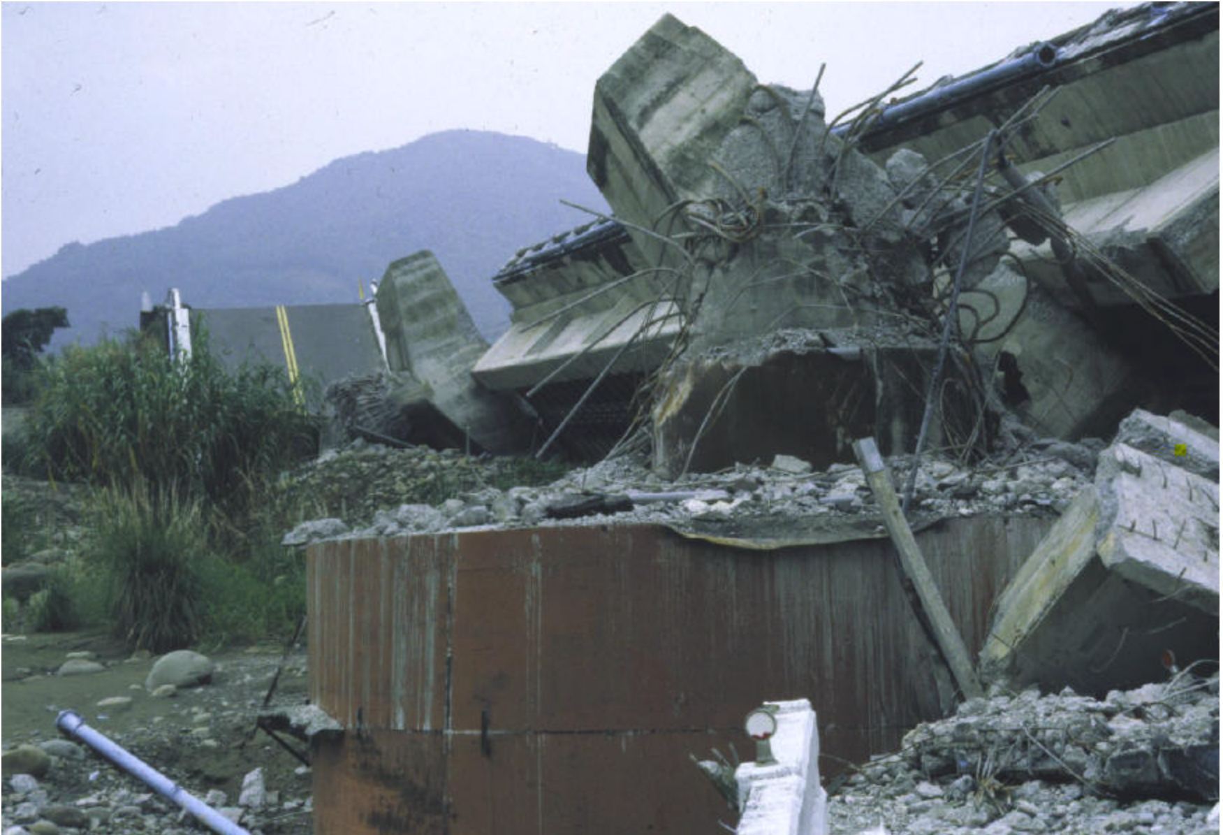
Toong-Tour Bridge, 921 Taiwan Eq. (1999) (M.O. Eberhard)
