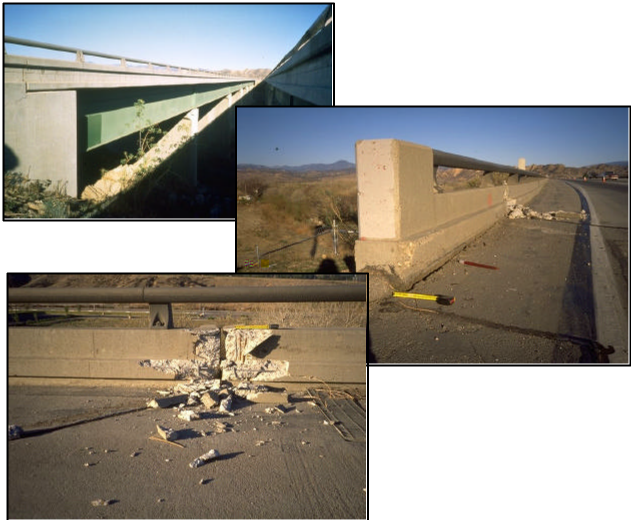
FIGURE 8.1 View of bridge superstructure after the earthquake (11)
