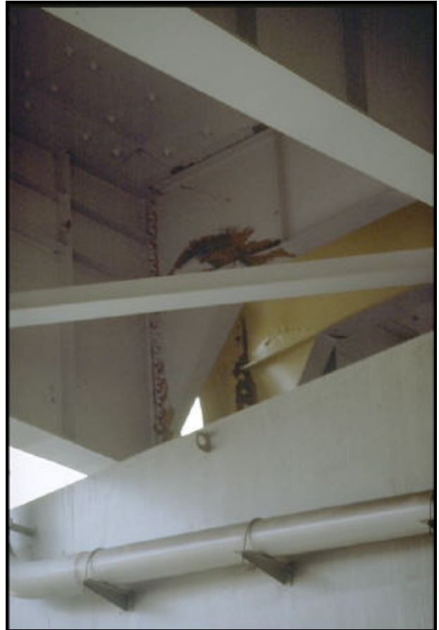
FIGURE 5.61 Local buckling of beam web near haunch (11)
