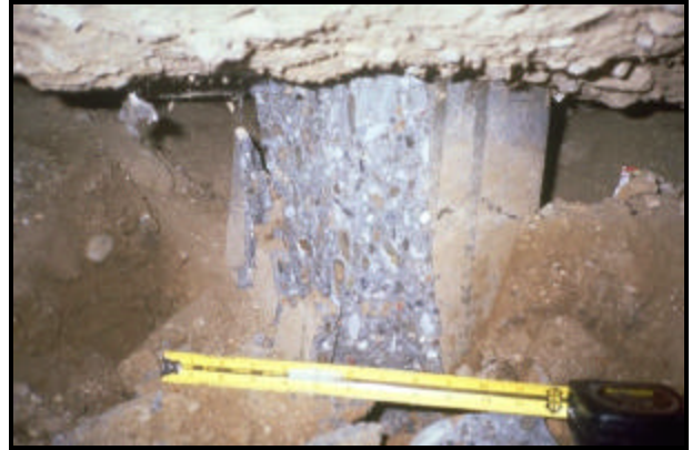
FIGURE 5.80 Spalling of concrete at the top of the pile for abutment after excavation (11)
