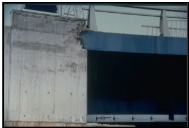
FIGURE 5.35 Pounding damage at abutment (11)
