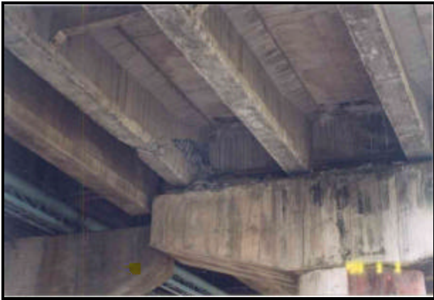
FIGURE 5.68 Shear cracks at the RC bridge girder near support (26)
