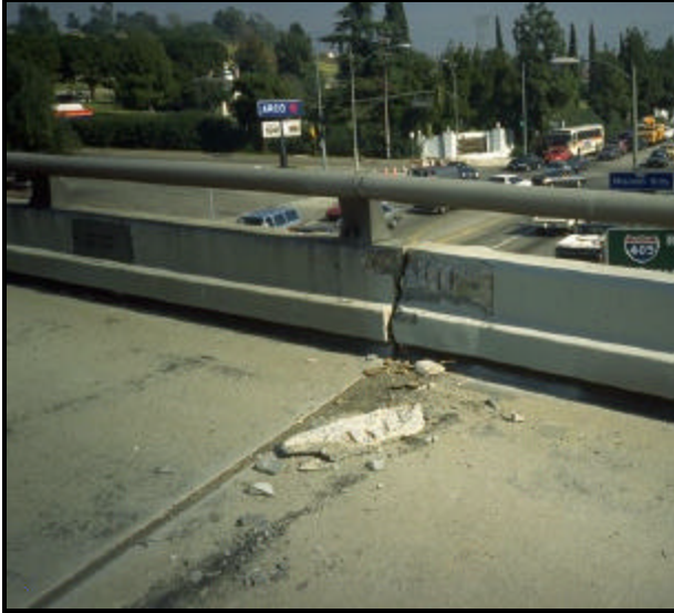
FIGURE 5.45 Minor damage on the deck of a bridge after Northridge EQ 1994 (11)
