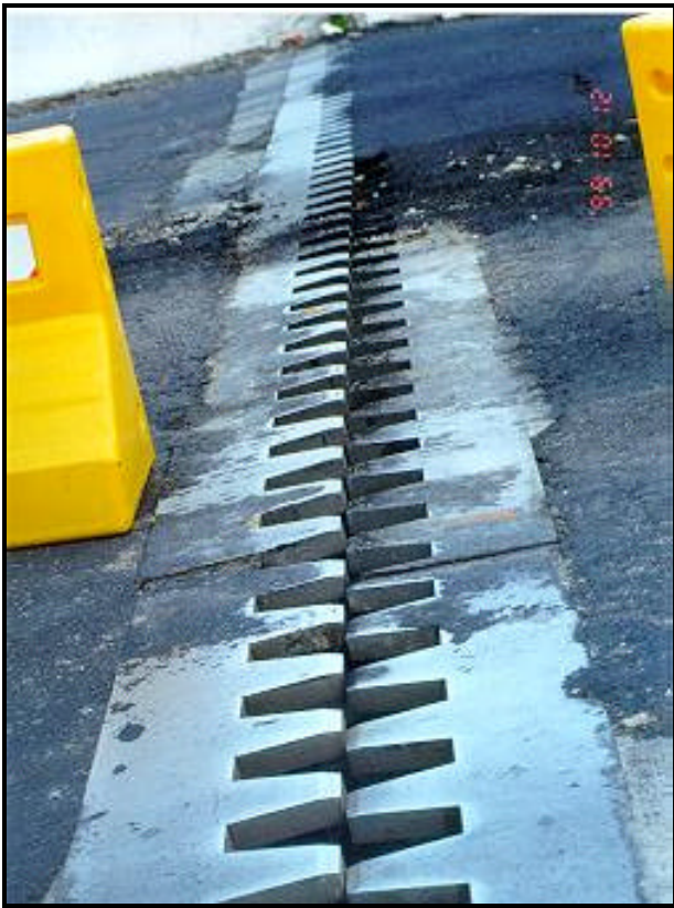
FIGURE 5.18 Excessive movement of expansion joints after Taiwan EQ 1999 (15)
