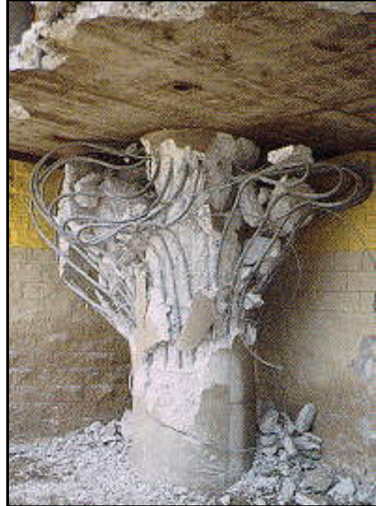
FIGURE 5.24 Failure of RC e column (11)
