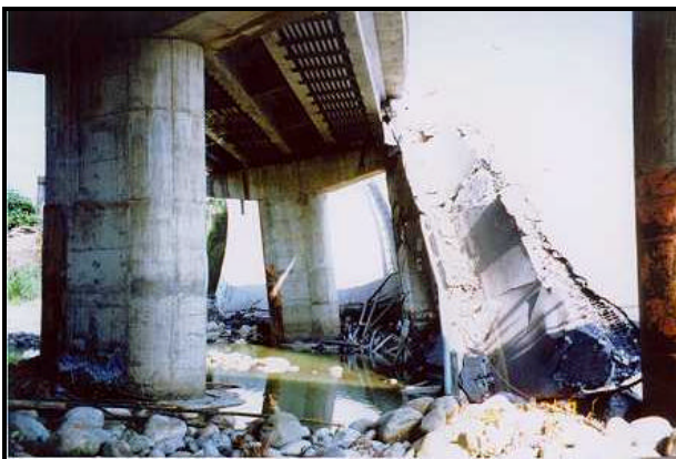
FIGURE 5.6. Collapse of deck and piers after Taiwan Earthquake 1999 (15)
