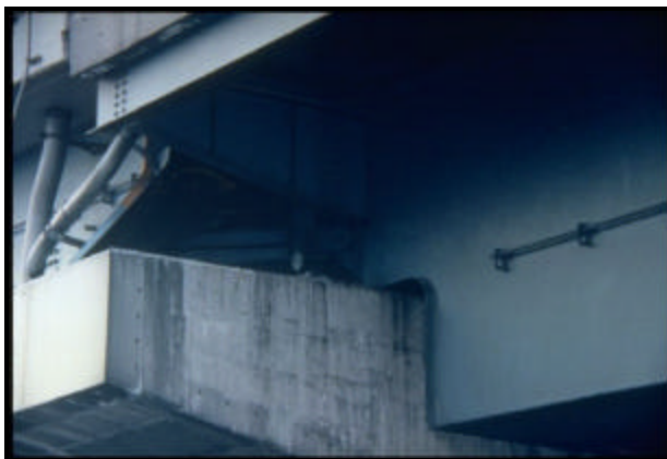
FIGURE 5.64 Steel box girder movement and collapse of bearings (11)
