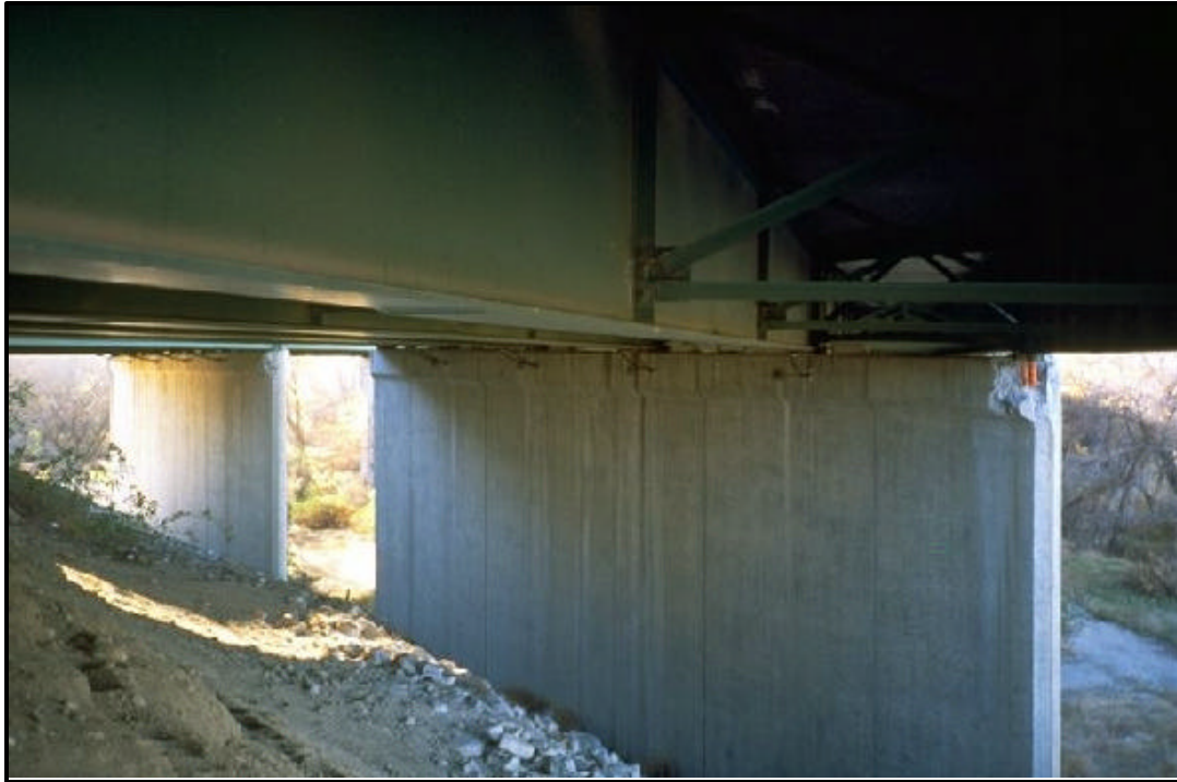
FIGURE 8.5 Damage to one of the bridge piers (11)
