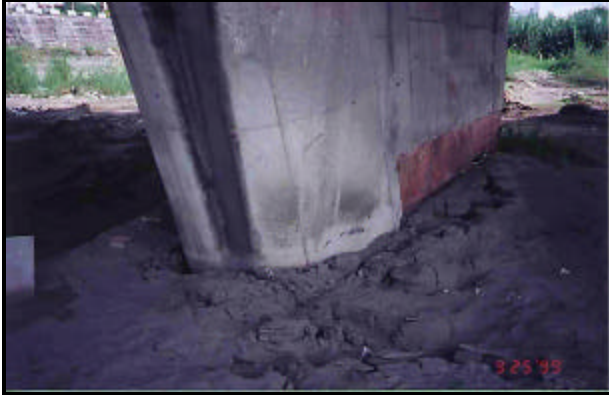
FIGURE 5.83 Ejected sand and lateral spreading around RC bridge pier (11)
