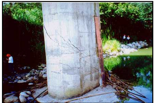
FIGURE 5.76 Heavily damaged RC bridge pier (15)
