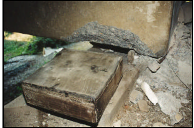
FIGURE 5.38 Failure of elastomeric bearing and cracking of girder beam (10)
