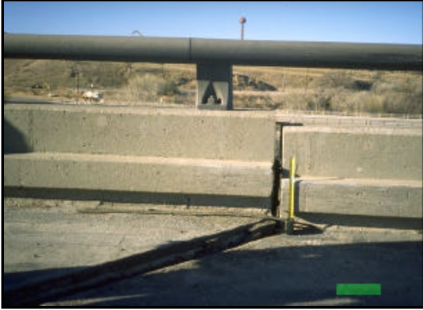
FIGURE 5.17 Vertical offset between decks after Northridge EQ 1994 (11)
