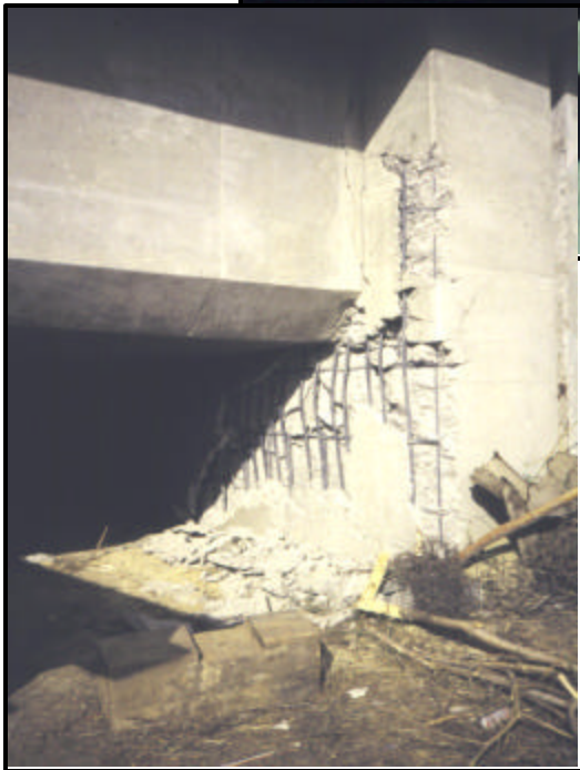
FIGURE 8.18 Different views of damage from the damaged bridge (11)
