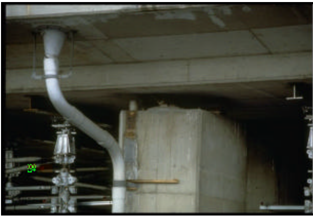
FIGURE 5.55 Shift of bearings after collapse (11)
