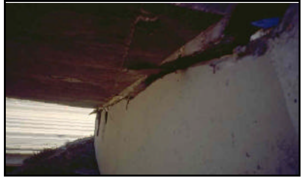
FIGURE 5.71 Separation of the RC superstructure and the abutment (11)
