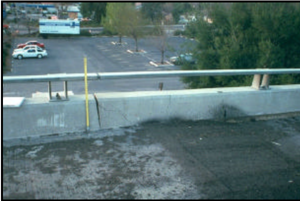
FIGURE 5.46 Curb separation after Northridge Earthquake 1994 (11)
