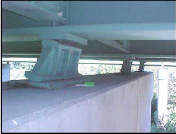
FIGURE 5.54 Tilted rocker bearings (9)
