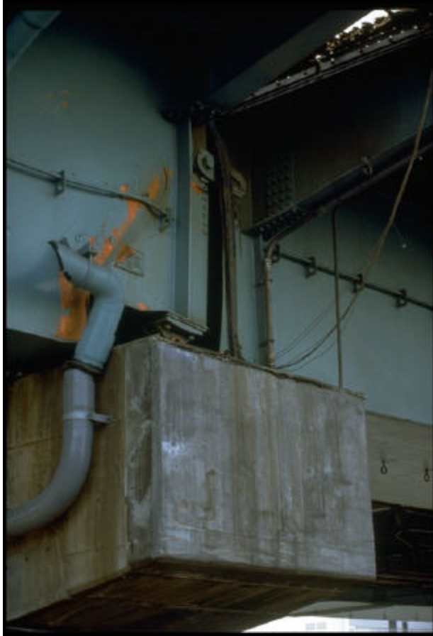
FIGURE 5.63 Buckling in the girder due to pounding (11)
