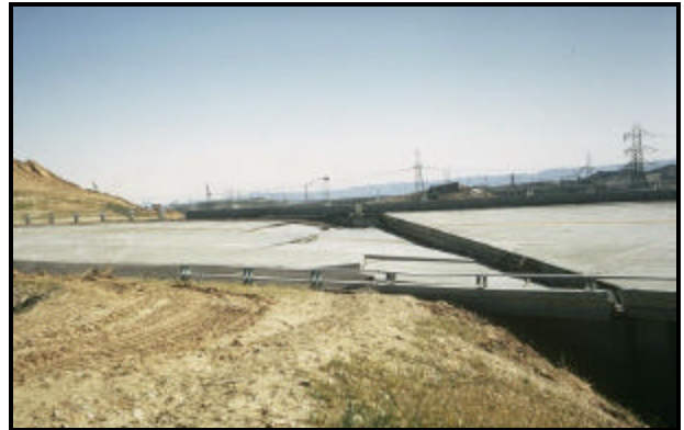
FIGURE 5.49 Settlement damage on approaches after Northridge EQ 1994 (11)
