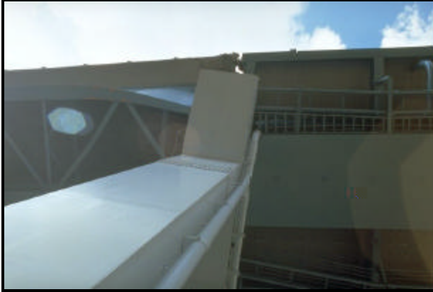
FIGURE 5.31 Buckling of steel girders (11)
