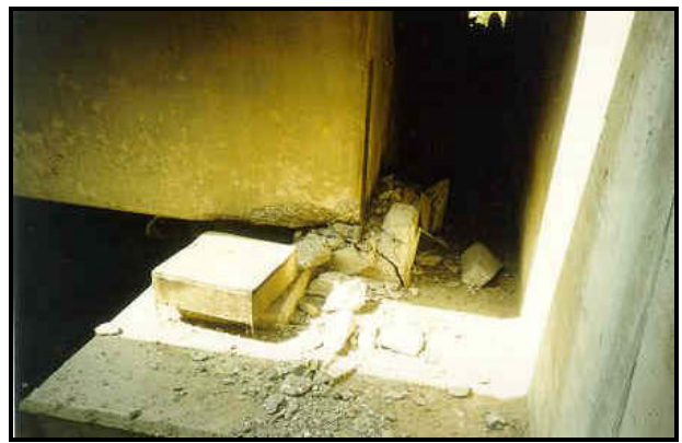
FIGURE 5.58 Sliding of elastomeric bearing (10)
