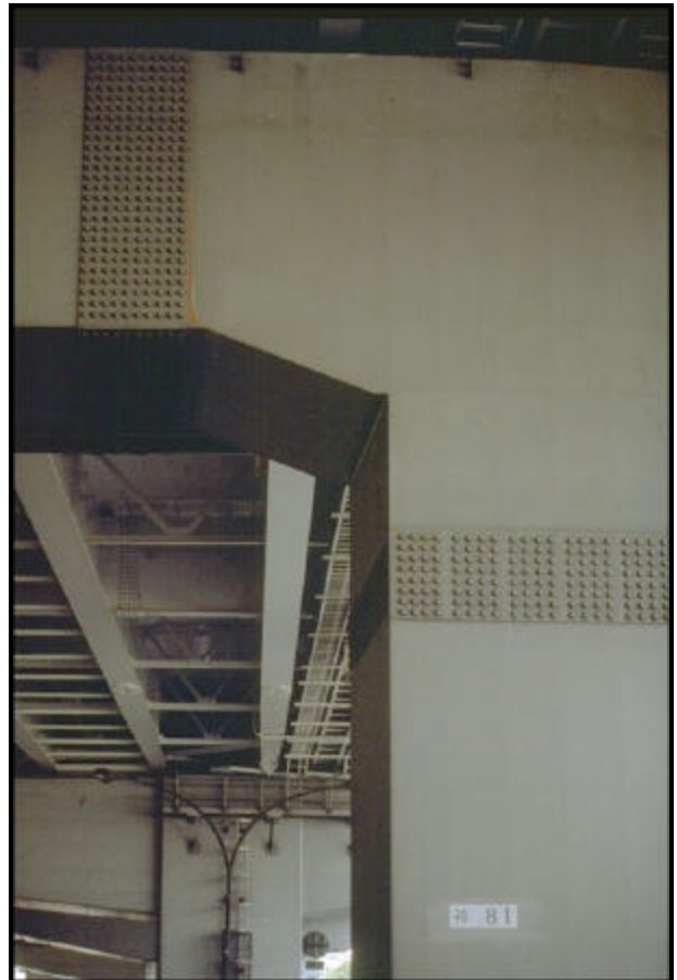
FIGURE 5.66 Yielding at bolted connector beam (11)
