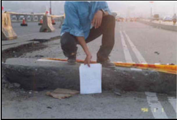
FIGURE 5.22 Settlement of Bridge (26)
