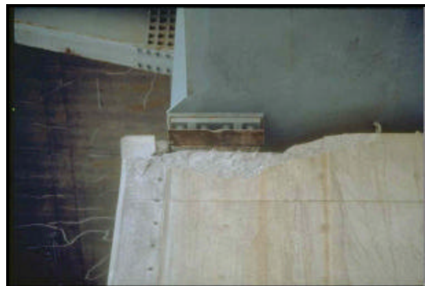
FIGURE 5.53 Bearing movement and concrete spalling on the pier (11)
