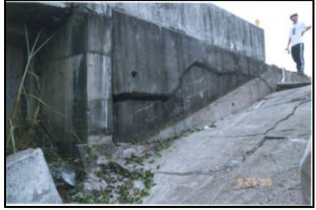
FIGURE 5.70 Large cracks at abutment wing wall and slope (26)
