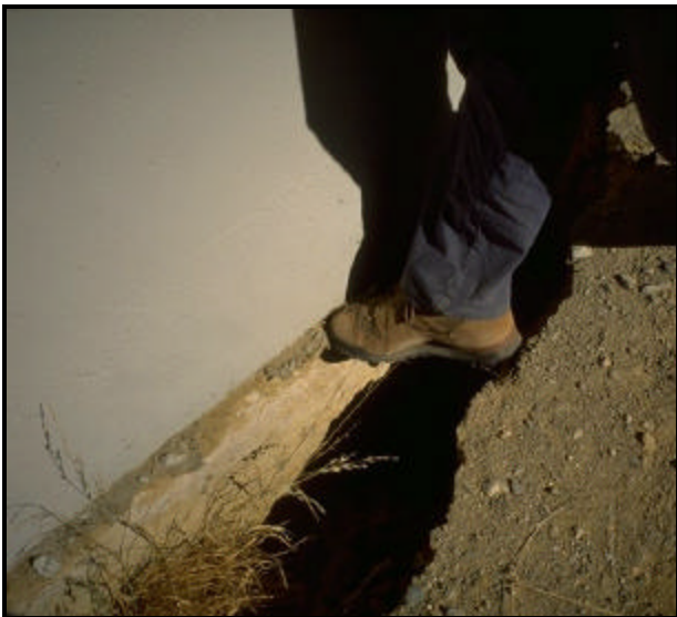
FIGURE 5.42 Separation of column from the surrounding soil after Northridge EQ1994 (11)
