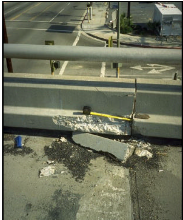
FIGURE 5.44 Barrier cracking after Northridge Earthquake 1994 (11)
