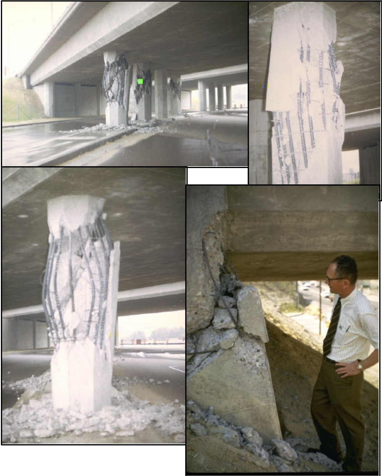
FIGURE 8.15 Substructure damage of the bridge (11)
