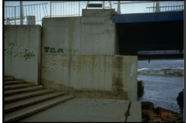
FIGURE 5.34 Transversal movement of abutment (11)
