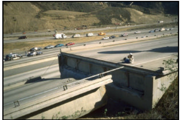
FIGURE 5.9 Collapse of bridge deck after Northridge 1994 (11)
