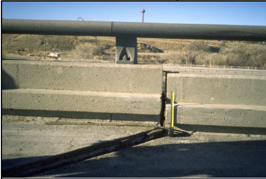
FIGURE 8.2 More damage to the bridge superstructure (11)
