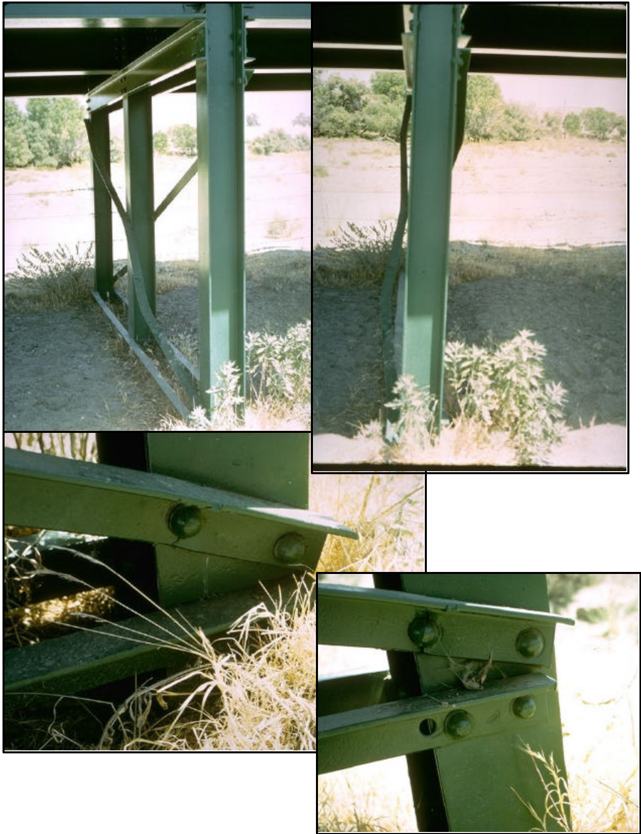
FIGURE 8.12 View of the damaged bridge components (11)
