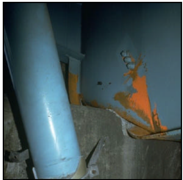
FIGURE 5.72 Pounding of steel girder to the abutment (11)
