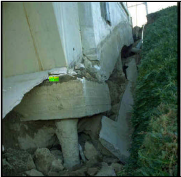
FIGURE 5.32 Movement of an abutment after Northridge Earthquake 1994 (11)
