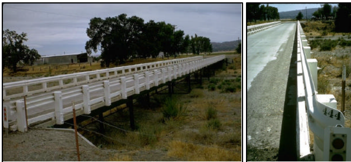
FIGURE 8.11 View of the Parkfield Highway Bridge after the earthquake (11)
