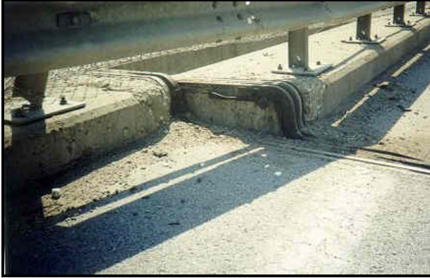
FIGURE 5.12 The excessive transversal movement of bridge after Izmit EQ (10)
