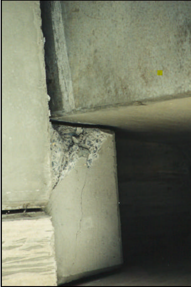
FIGURE 5.73 Concrete spalling and cracking due to pounding of RC box girder after Izmit EQ 1999 (10)
