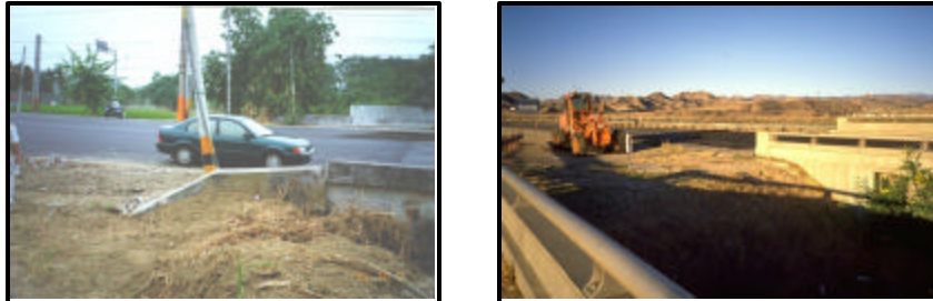
FIGURE 7.2 Different bridge damage cases that fill can be used (15,11)
