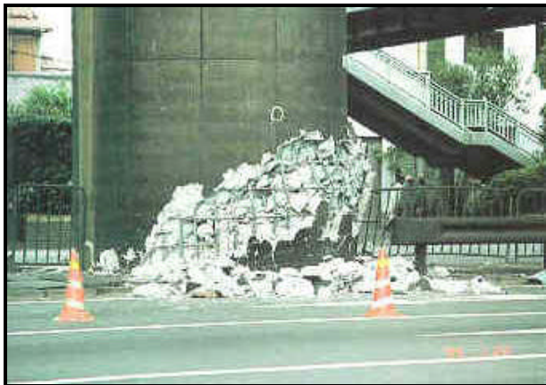
FIGURE 5.27 View of damaged RC bridge pier after Kobe Earthquake 1995 (13)
