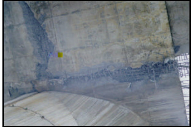
FIGURE 5.65 Heavy damage in RC box girder bridge (15)
