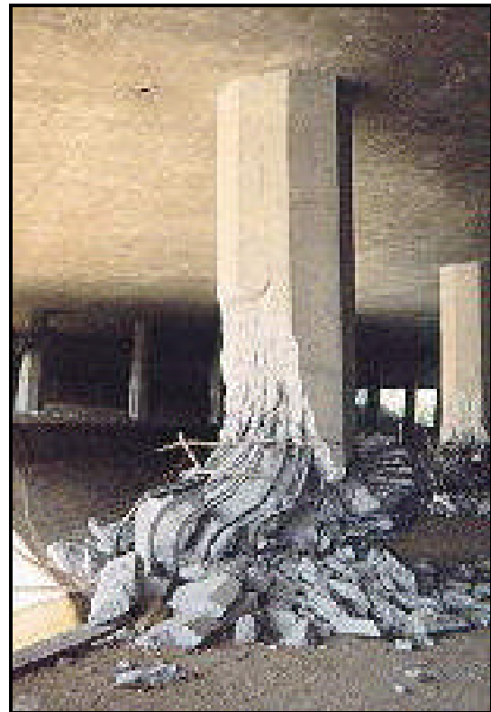
FIGURE 5.25 Failure of the bottom of the RC bridge column (11)
