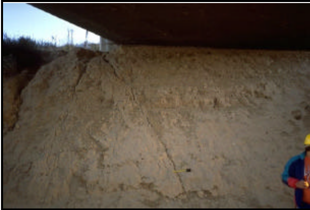
FIGURE 5.77 Ground crack extending diagonally down slope under bridge (11)
