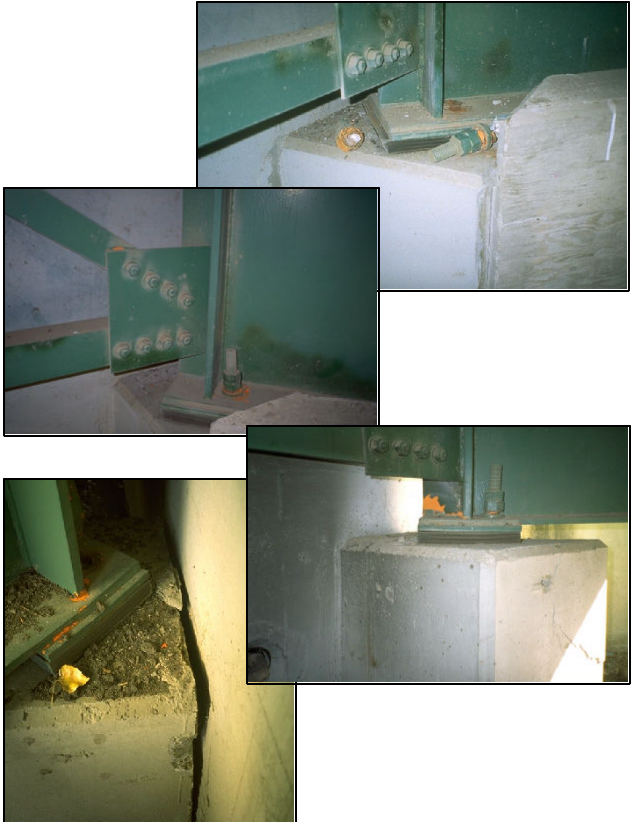
FIGURE 8.7 Damage to the bridge bearings (11)
