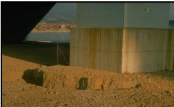
FIGURE 5.79 Settlement around RC bridge pier (11)
