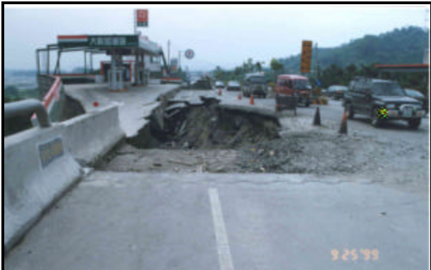
FIGURE 5.69 Abutment slumping after Taiwan EQ 1999 (26)
