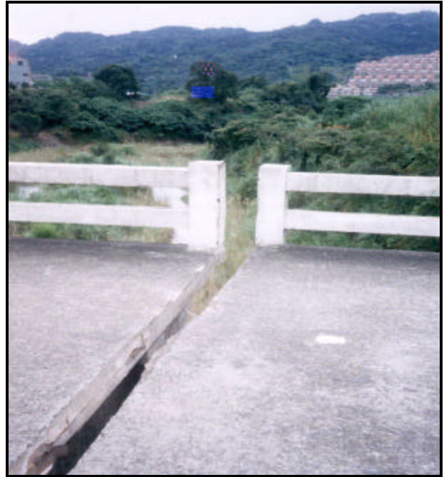
FIGURE 5.11 Excessive longitudinal movement of the bridge deck (15)
